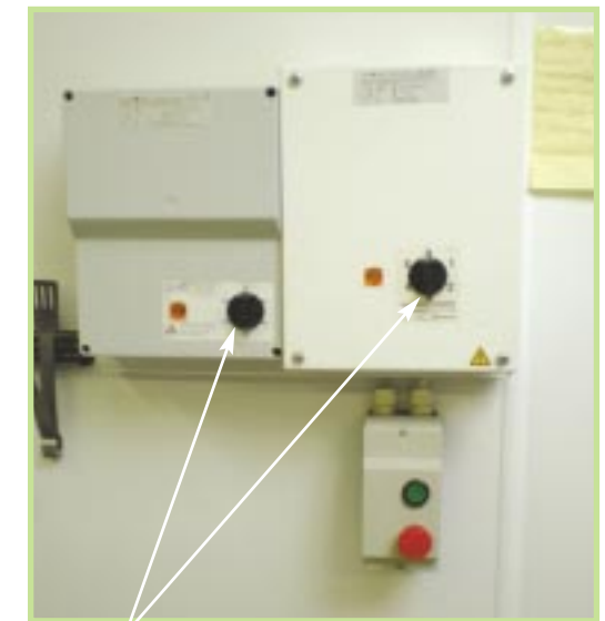
Variable speed drives can reduce energy consumption for extractor fans
