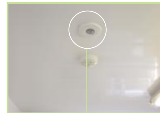
Motion sensor which turns on light automatically
