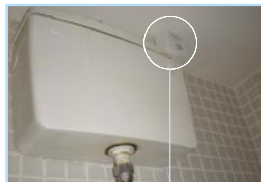
Motion sensor which has been retrofitted to urinals to conserve water and save
