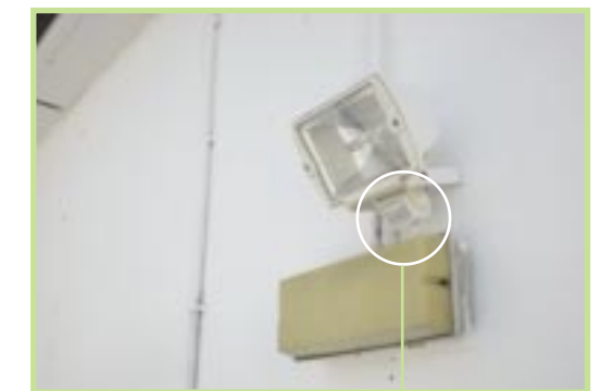
Motion sensor to activate security lighting
